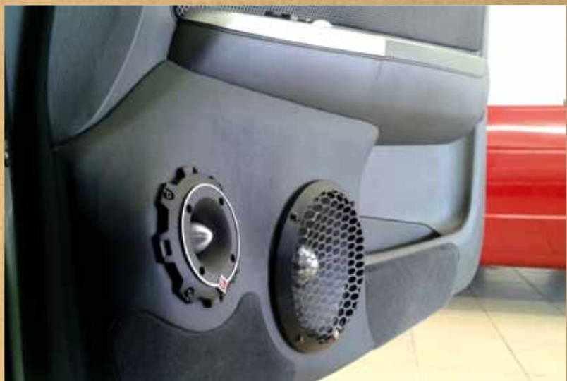
ICE specialists, Cellsound, will handle the installation of the sound system. Custom door panels will look something like this...
