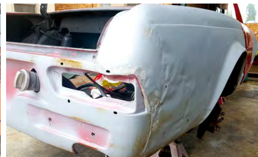
On arrival this Merc Pagoda didn't look bad, but the stripping process uncovered thick layers hiding poor past repairs. This is the back corner and the front right is not much better. Before progressing, the unsuspecting client will be shown and a game plan to do it right made.
